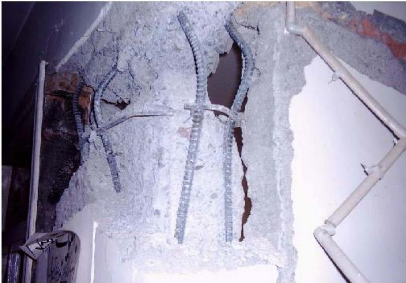
Figure 7: Formation of plastic hinge in the column near the beam-column joint in a hospital building in Mansehra
